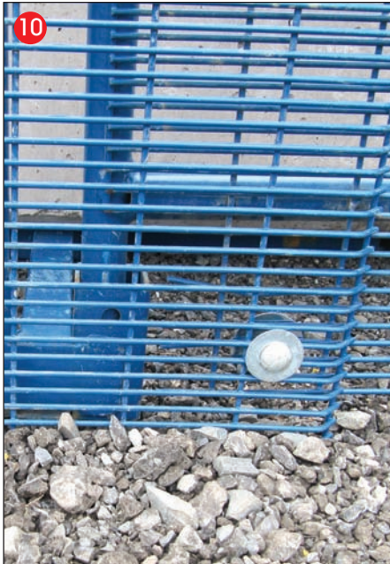
Bottom Cover Mesh bolt to be no more than 50mm from ground.
